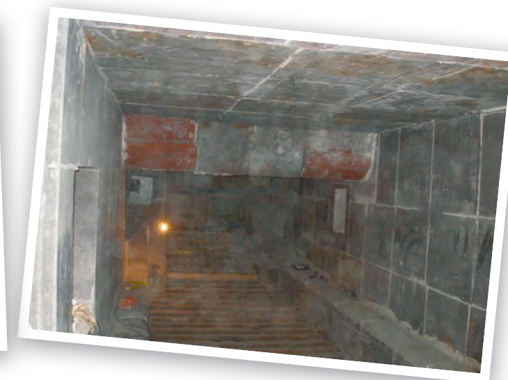
Casted grate cooler, Greece
