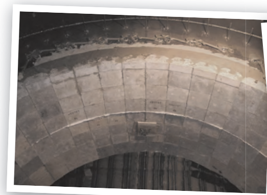
Kiln hood in precast shapes, Germany
